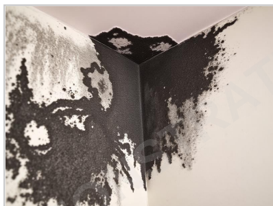
Photo 1 — Rear Bedroom 2 Severe recurring black mould at corner junction of external walls in rear bedroom
