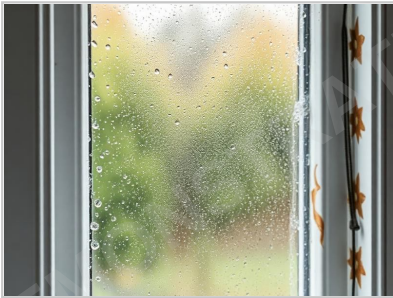
Photo 1 — Kitchen/Diner Heavy condensation streaming on kitchen window with early mould on frames
