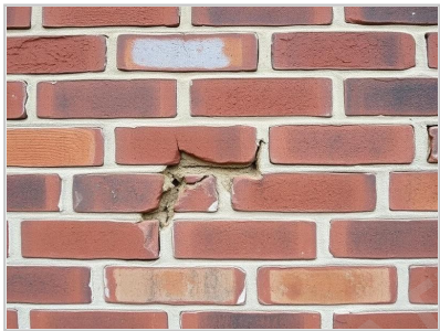
Photo 1 — Pointing & Mortar Joints Deteriorated pointing to front elevation with recessed mortar joints Photograph taken at time of inspection. Photographs taken at time of inspection.
