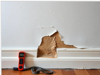
Photo 1 — Rear Reception Room Rising damp tide mark with salt deposits on rear reception wall
