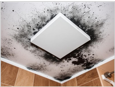
Photo 1 — First Floor Bathroom Black mould growth on bathroom ceiling around extractor fan Photograph taken at time of inspection. Photographs taken at time of inspection.
